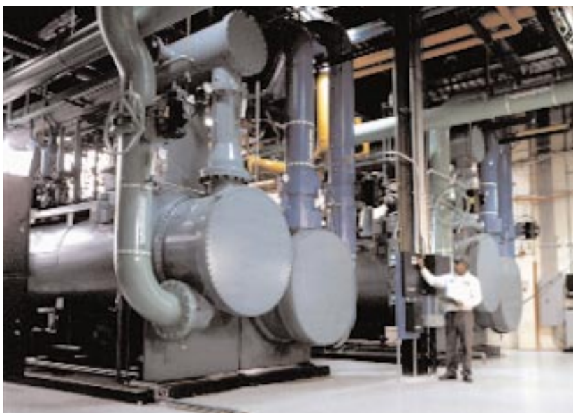
Shown are the two 1200-ton, steam-turbine-drive, HFC-134a, centrifugal chillers. The condensate systems are installed above the chillers in order to meet space constraints.
