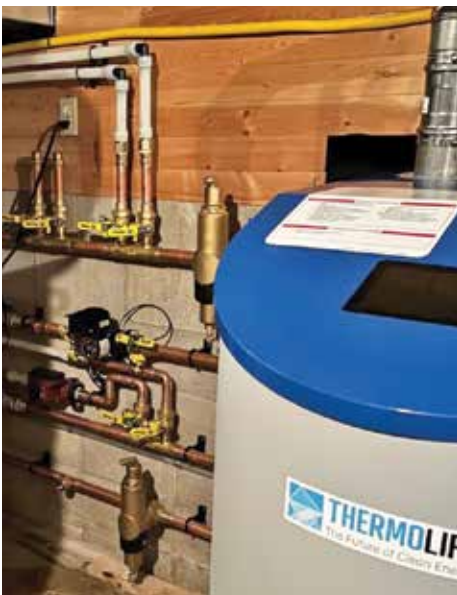
PHOTO COURTESY OF THERMOLIFT INC.
